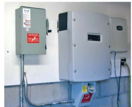
PV power inverter installed by Jim Dunn.
