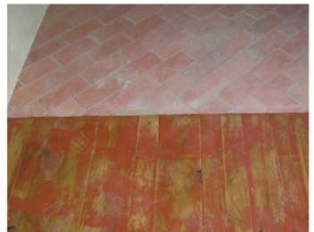
All flooring is either brick or hardwood. Radiant tubing is embedded under the brick. Ecowarm™ radiant floor panel was used under the hardwood floors.
