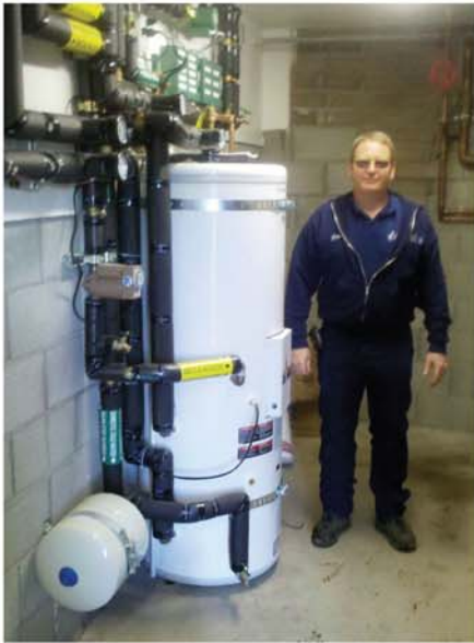
Mechanical contractor John Lockwood standing next to Daikin's indirect water heater with supplemental electric backup.
